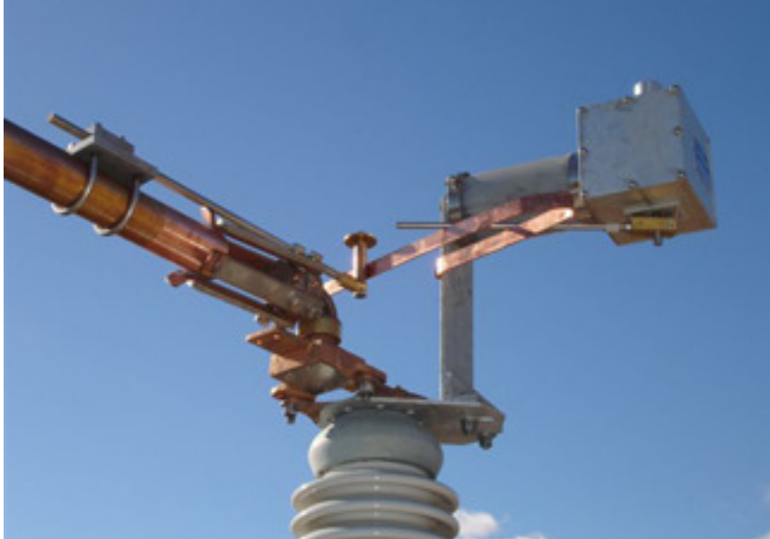
Type SM single bottle interrupter on a 138 kV side break switch
